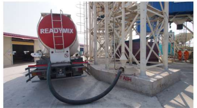
Transfer of fly ash from Readymix Tanker to silos through pneumatic blower to a pipe mounted on the side of silo
