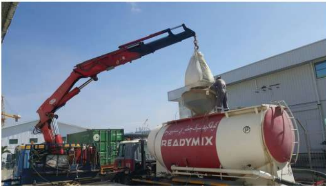
Loading of fly ash into Readymix tanker and thereafter to be pump into silo
