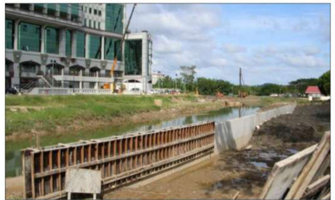
Gadong Drainage system (BSB)
